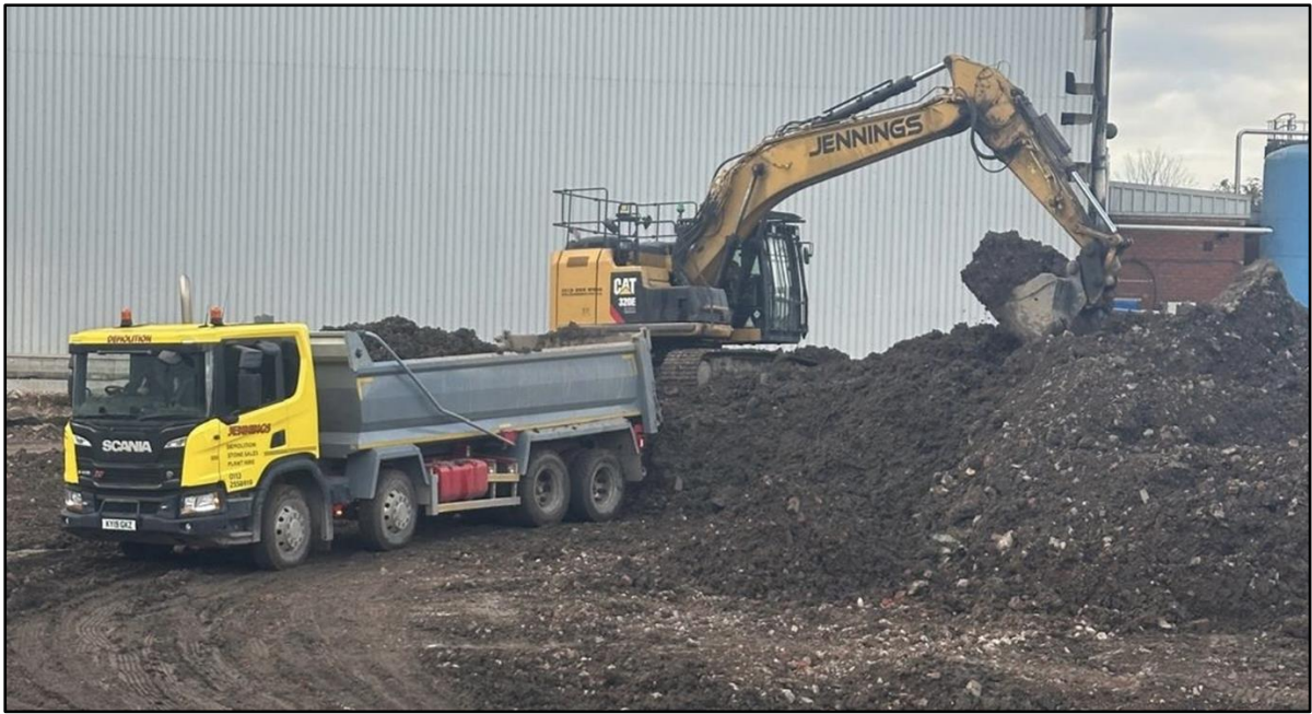
Figure 12: Image showing excavated material being loaded onto a lorry for removal from site, due to a lack of on-site storage space (Photo by the author, 2024).
